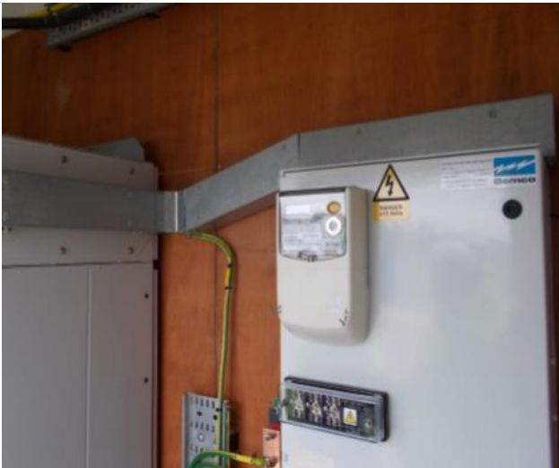
BEFORE (In need of rectifying)
